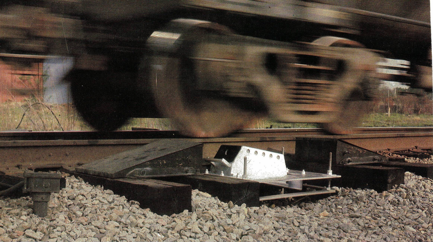
Hybrid, microprocessor-upgraded Servo detector installation on the Seaboard System at Goose Creek, S.C. scanning journals on a passing freight. Current railroad wayside defect detection programs include such enhancements as updated scanner monitoring and electronics, on-site heat-signature processing on the basis of refined alarm criteria, data digitization for transmission, and direct radio "talker" identification to train crew members of multiple types and locations of detected defects.
